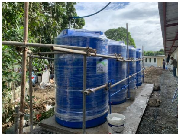
Water supply tanks
